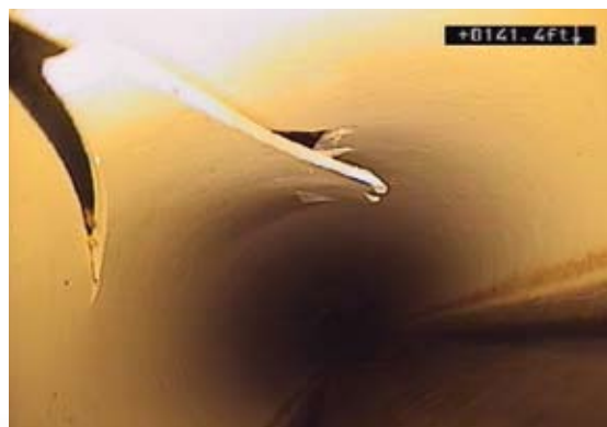
SEWER LINE BEFORE CIPP POINT REPAIR
