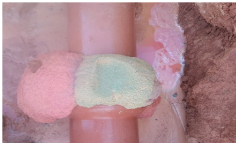
Figure 158: Red and Blue Grout Separated
