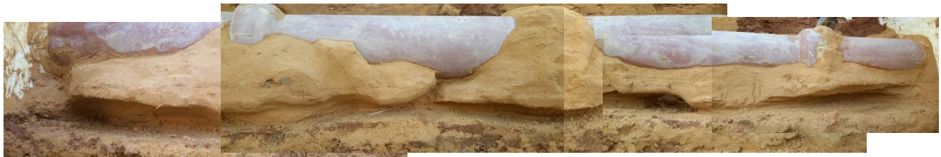
Figure 78: Close-Up of Lower Portion of Defect Seals and Pipe Stabilization
