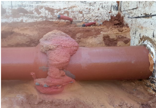
Figure 38: Defect C Seal Side View
