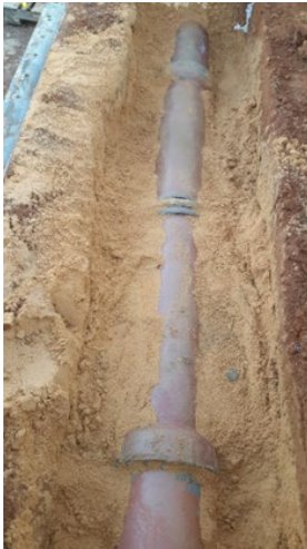
Figure 89: Pipe with Defects Installed
