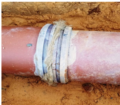
Figure 10: Defect B - Full Circumferential
