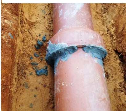
Figure 9: Defect C - 12 o'clock Position
