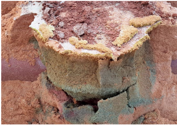
Figure 58: Upward Grouted Mass Above Defect
