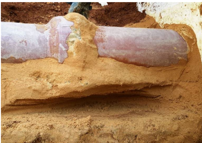
Figure 68: Grout Migration Below Pipe
