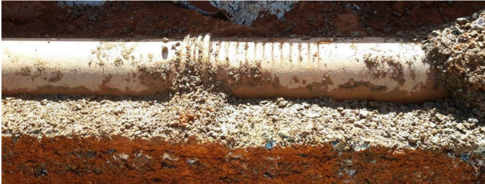
Figure 174: Defect A at 3 O'clock Position Grouting in Stone
