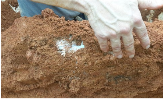
Figure 141: Fin Origin at Defect
