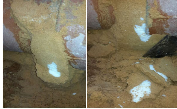
Figure 101: Neat Grout Lens Observed
