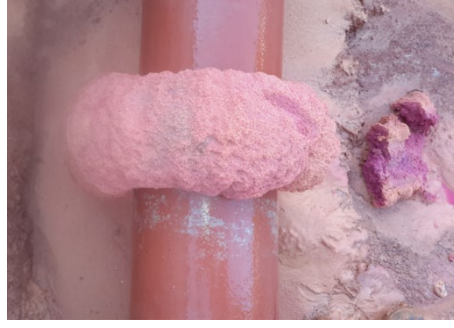
Figure 33: Defect B Formation Top View
