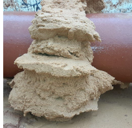
Figure: 138: Defect B 23 Second Gel Time
