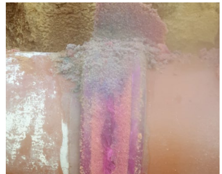
Figure 37: Defect B Removal of Top Seal
