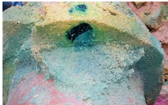
Figure 187: Defect C Grout Seal (12 O'clock)
