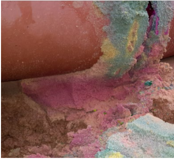
Figure 43: Red Grout Observed Below Pipe
