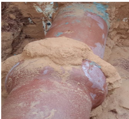
Figure 99: Seal at 12 O'clock Position
