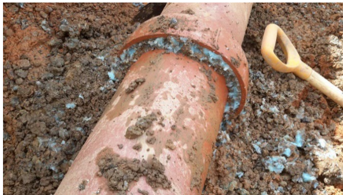
Figure 127: Grout Filled Circumferential Defect B
