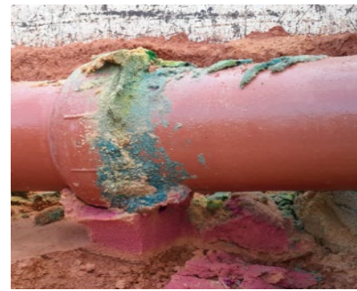
Figure 50: Dissection of Defect C
