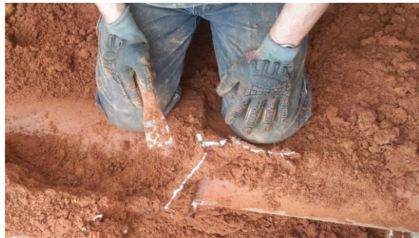
Figure 175: Grout Fin Extending from Defect
