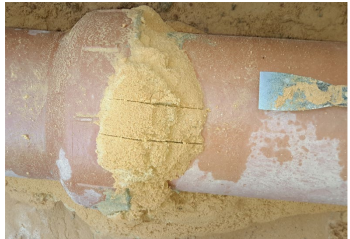
Figure 69: Top View Grouted Defect
