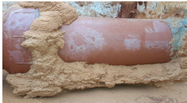
Figure: 100: Observed Longitudinal Support of Pipe
