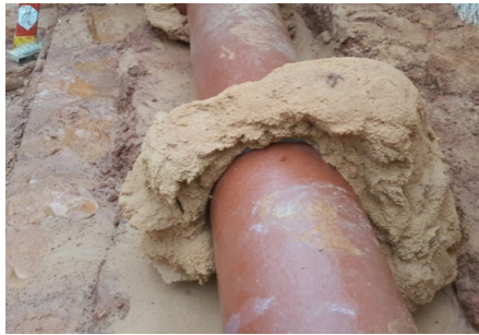
Figure 94: Side view of grouted defect
