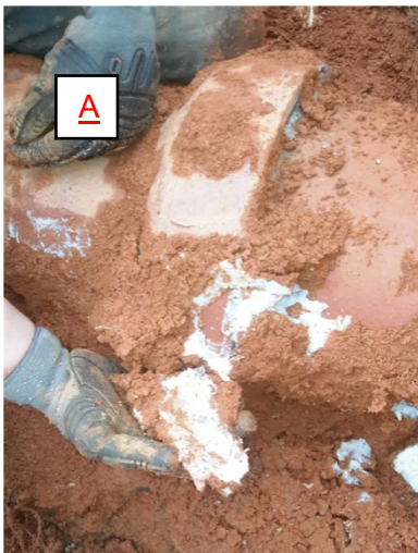
Figure 152: Defect A Seal
