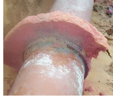
Figure 34: Defect B Side View
