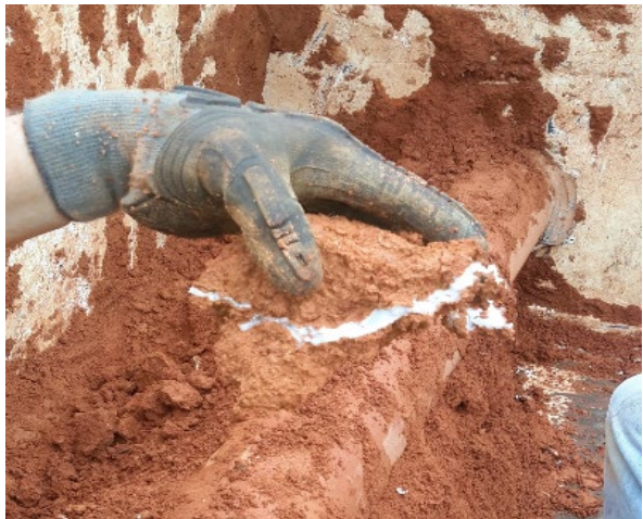
Figure 176: Neat Grout Fin
