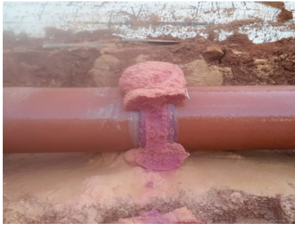
Figure 32: Defect B Grout Formation
