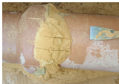
Figure 87: Defect Seal at 12:00 Position
