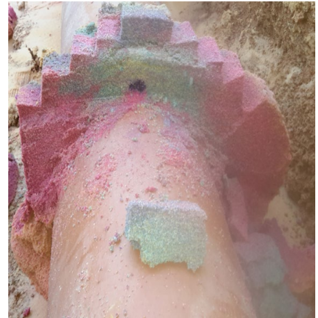
Figure 42: Defect C Neat Grout Seal Exposed
