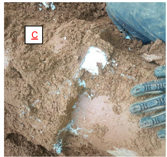
Figure 154: Defect C Seal
