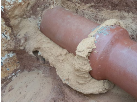
Figure 97: Sealed Joint with Pipe Support
