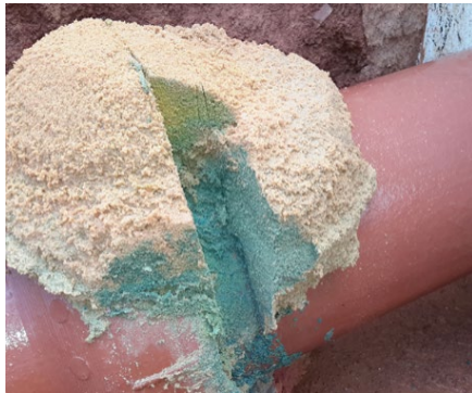
Figure 46: Dissection of Defect C
