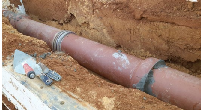
Figure 115: Joint Defect Prior to 57 Stone Installation
