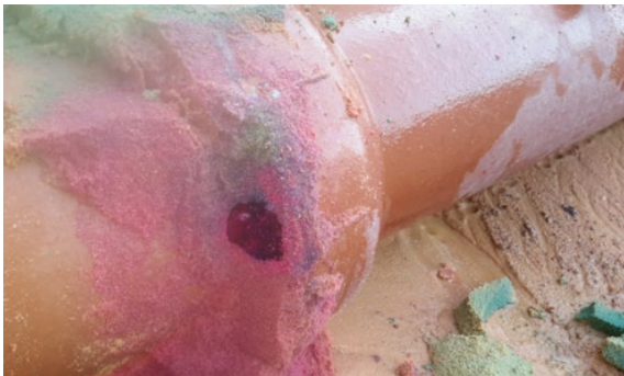
Figure 186: Defect A Grout Seal (3 O'clock)
