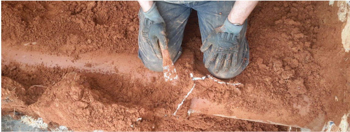
Figure 145: Fin Origin at Defect
