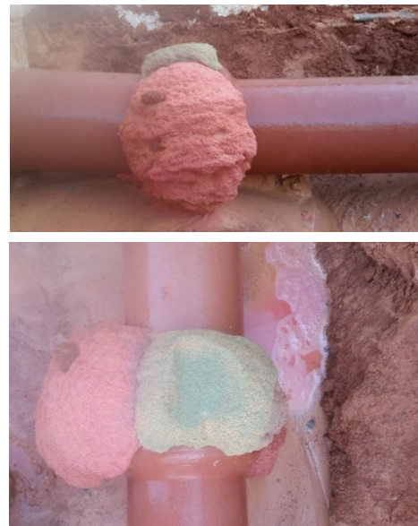
Figures 25 & 26: Defect A Observation
