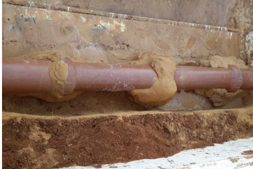
Figure 76: Top / Plan View of Grouted Defects
