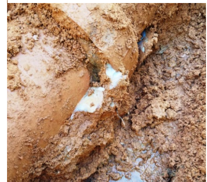
Figure 138: Seal at Defect
