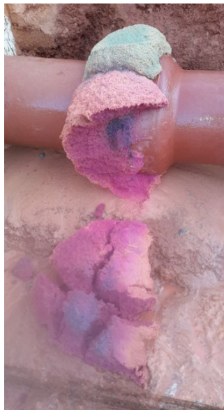
Figure 24: 2 Distinct Colors Observed at Defect A
