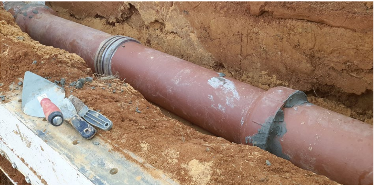
Figure 8: Pipe Defects Recreated Prior To Backfill
