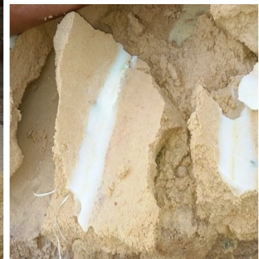
Figure 75: Voided Area Below Pipe
