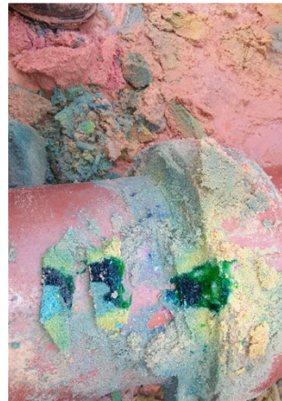
Figure 53: Neat Grout at Center of Defect
