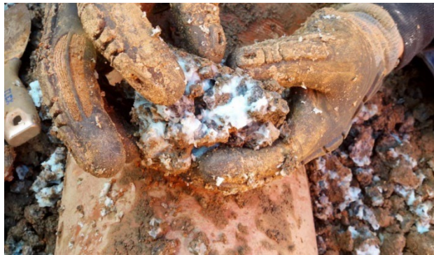
Figure 119: Pockets of Neat Grout
