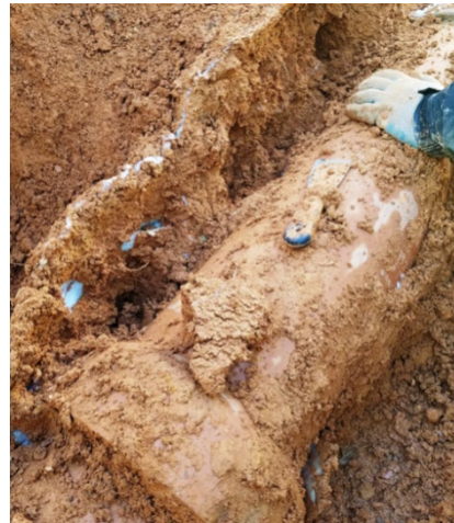
Figure 137: Fins of Grout
