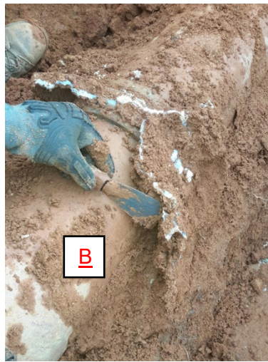
Figure 153: Defect B Seal
