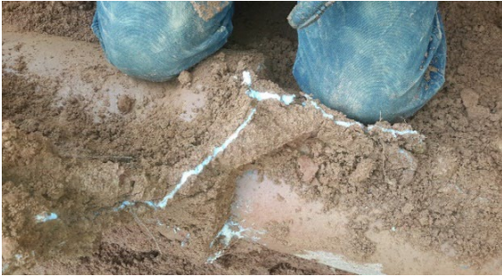
Figure 150: Exposing Defect and Seal
