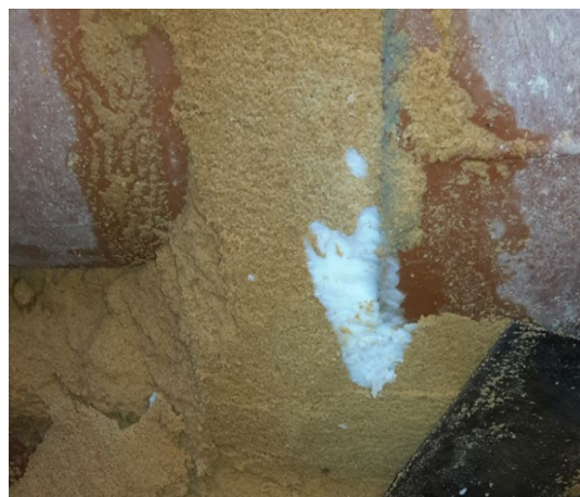
Figure 189: Neat Grout Located at Defect
