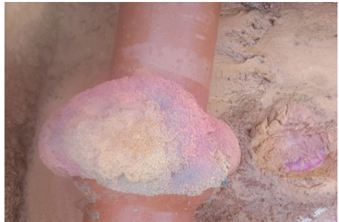
Figure 39: Defect C Seal Top View
