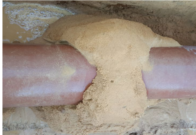
Figure 71: Top View Grouted Defect
