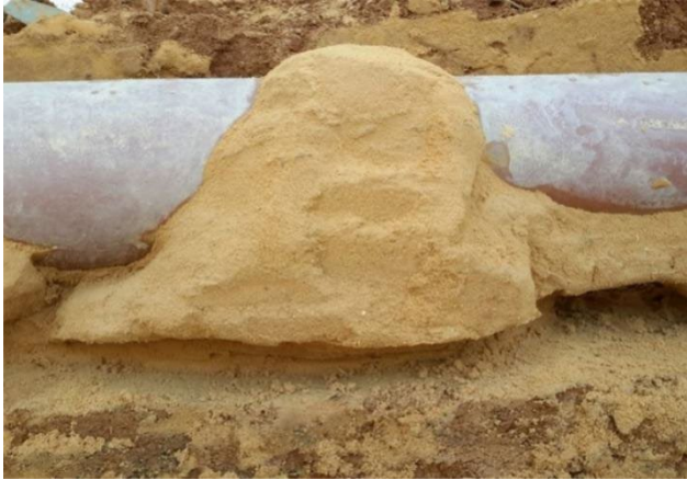
Figure 70: Side View Grouted Defect
