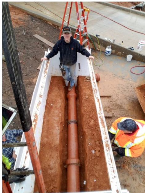
Figure 6: Pipe Install with Defects
