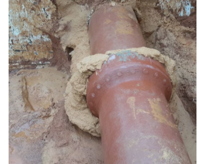
Figure 98: Grout Matrix observed on opposite side of defect.
