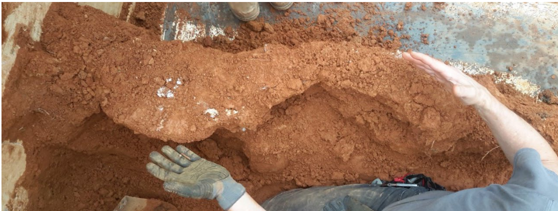
Figure 144: Further Observation of Grout Fins
