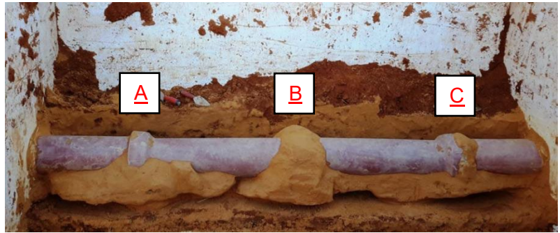
Figure 77: Side View of Grouted Defects A, B, & C
