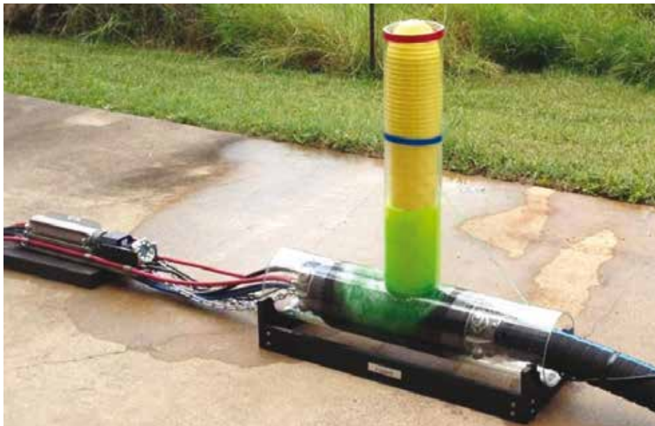
Facing page: Workers install Logiball's 108-inch main line packer at a job in Granite City, IL, where seasonally high groundwater has had a negative effect on underground facilities. A large sewer rehabilitation project rehabilitated 15,600 lineal feet of concrete pipe ranging from 72 to 108 inches in diameter.
