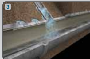
Continues to leak in annular space
