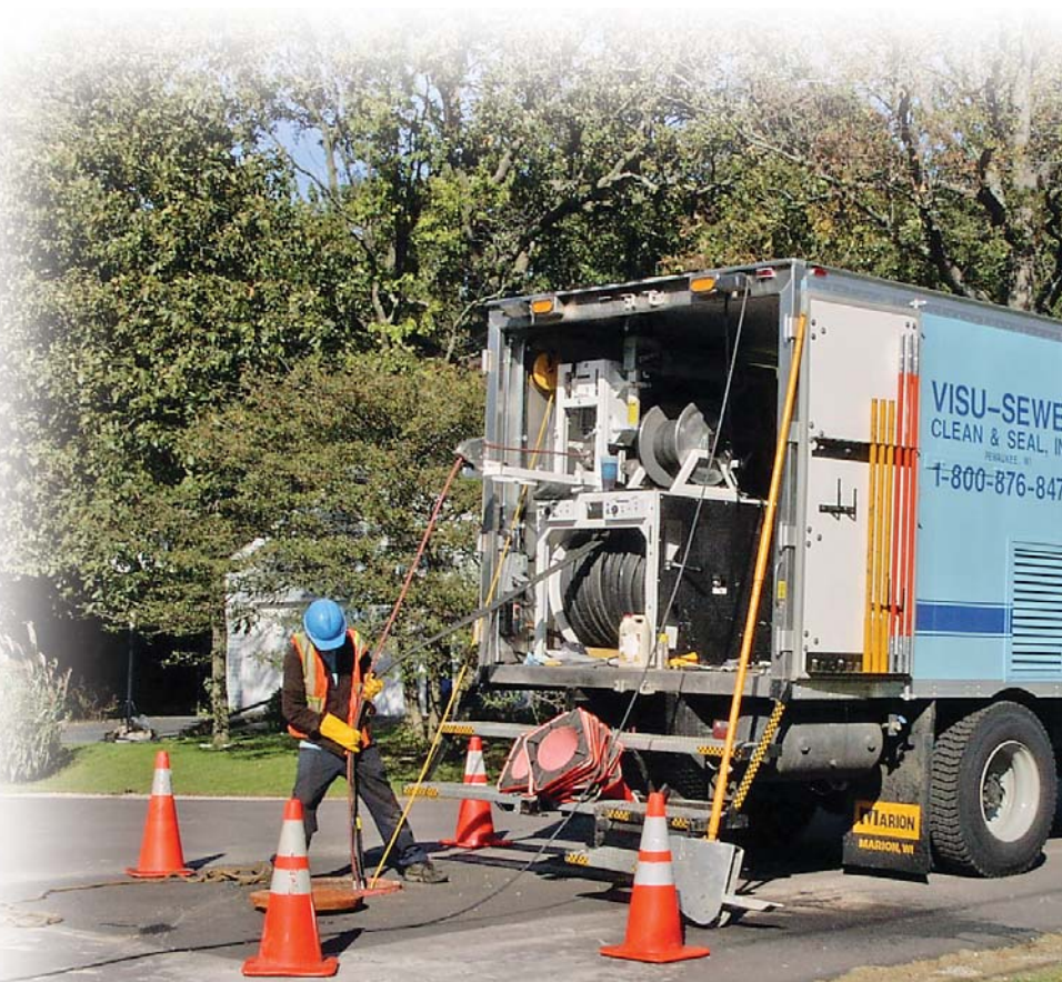
A technician from Visu-Sewer Clean & Seal Inc. starts an inspection of a sewer main in the City of Graettinger, Iowa, as part of the city's program to control inflow and infiltration.
