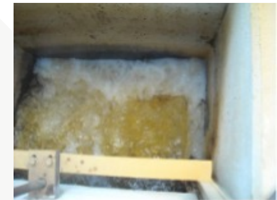
Figure 1. High-flow, high-turbulence areas like this flash mixer face increased corrosion potential due to high levels of H 2 S gas that deposits on surfaces.
