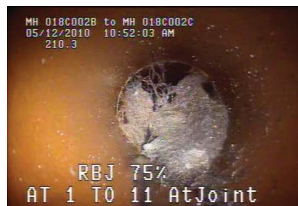
Root Ball Joint in Sanitary Sewer Photo Credit: NASSCO PACP Manual v.8.0
